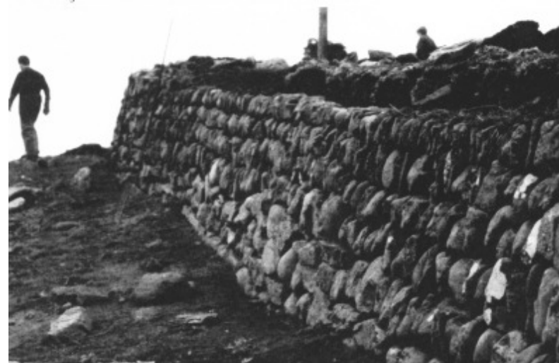
Clawdd built by trainees at Cemlyn, Anglesey, showing an amount of variation in the coursing
